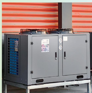
Outdoor Integrated Unit – Actual Photo
